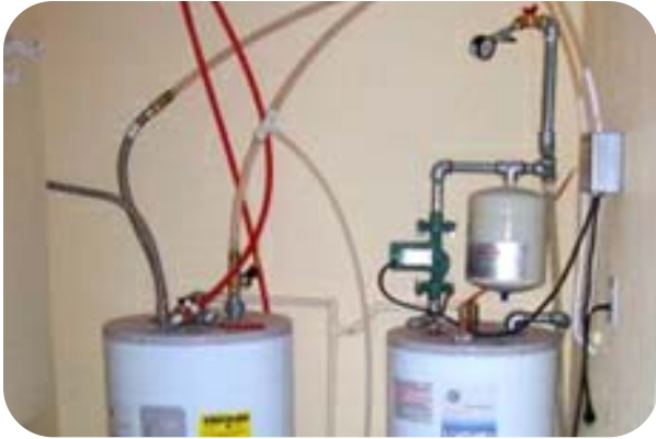
Heat Exchanger in Shed ©Melinda Honn
